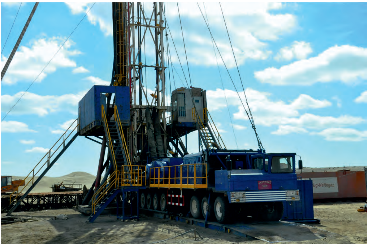
Goturdepe oilfield: Side-tracking by using ZJ-40 mobile drilling rig (225 ton load capacity)
