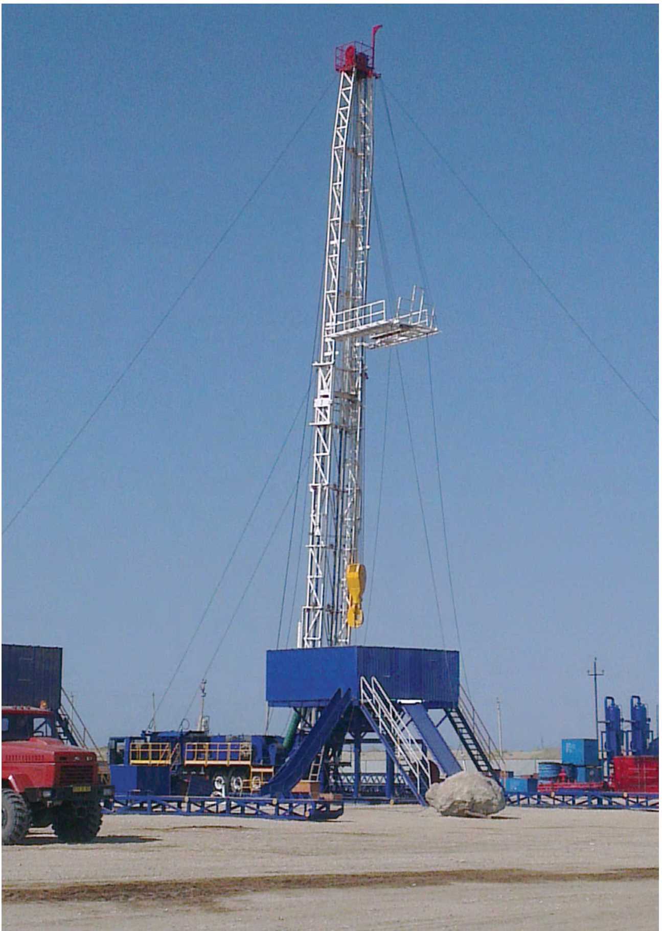
Barsagelmez oilfield: Well workover job in abnormal operating conditions by using ZJ-40 mobile drilling rig (225 ton load capacity)
