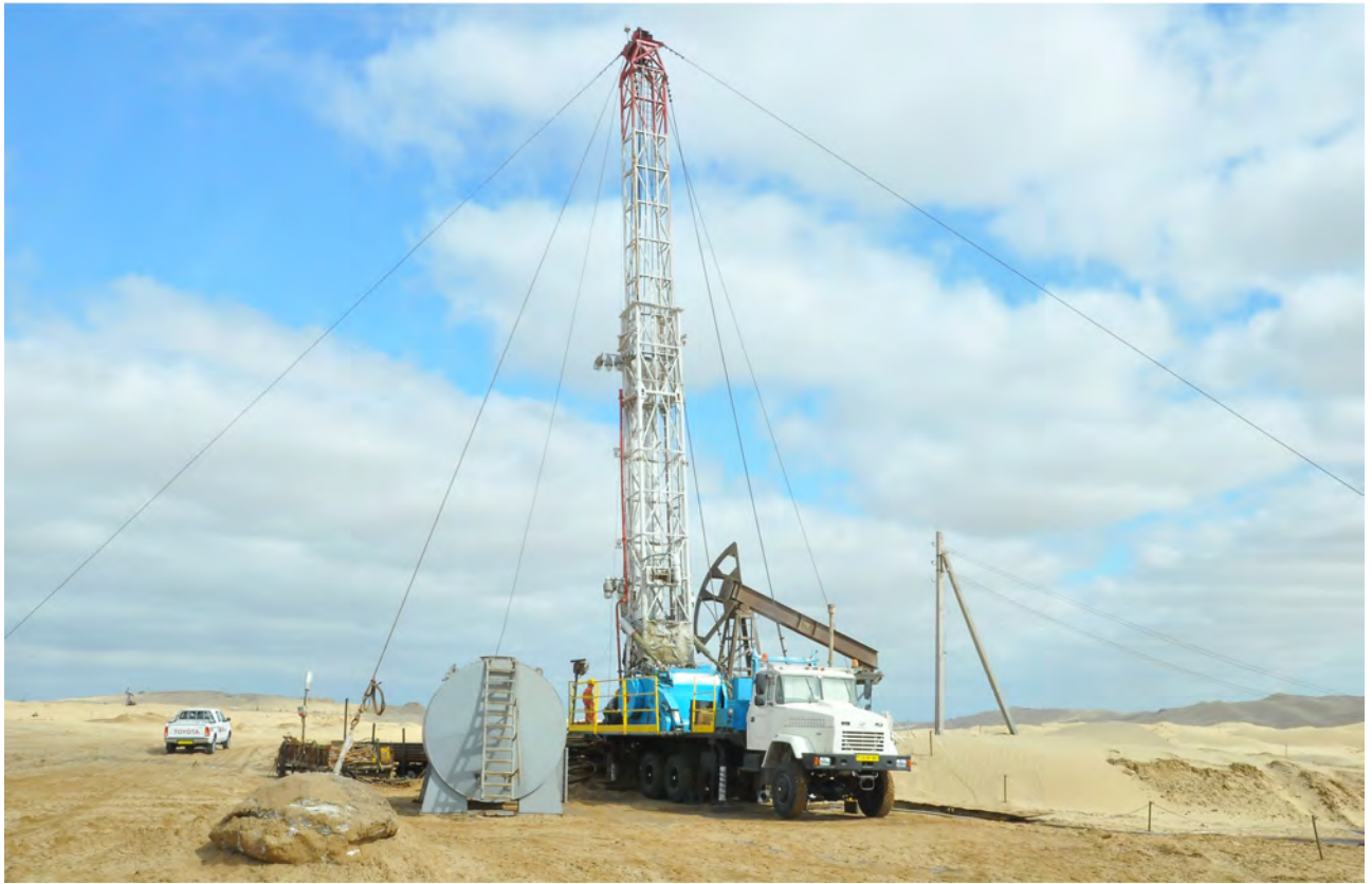
Goturdepe oilfield: Water shut-off jobs by using a workover rig (80 ton load capacity)
